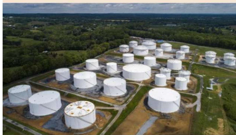
Colonial pipeline fuel tanks in Woodbine, Maryland (EPA)
